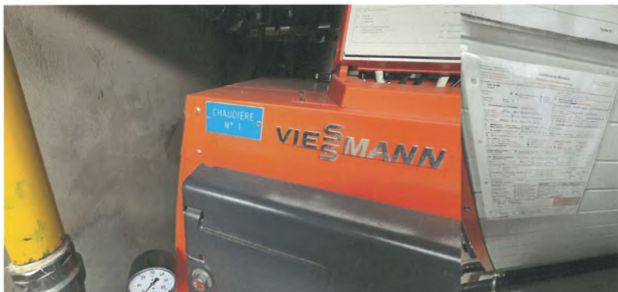
Figure 17 : Chauffage Haus am Becheler
