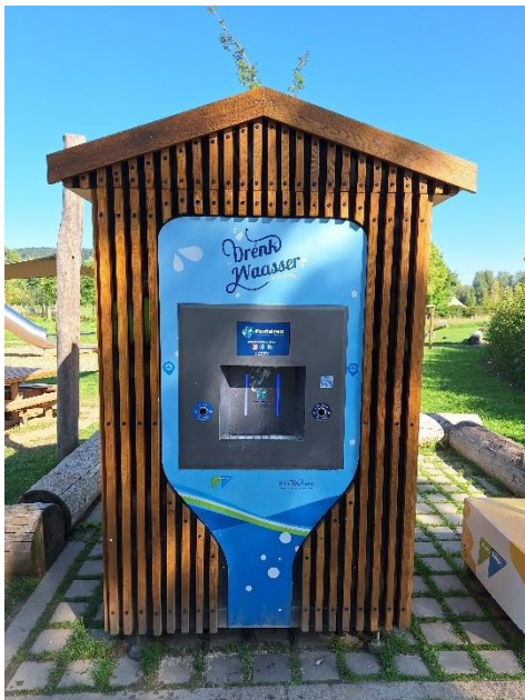
Trinkwasserstation in Helmsange
